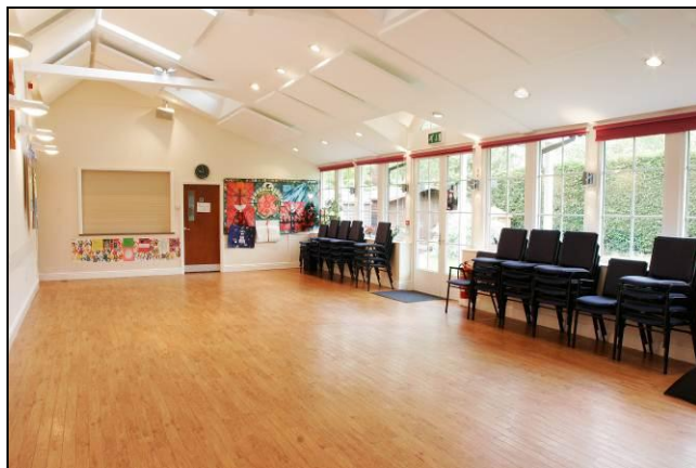
Sonata Vario installed to the ceiling at Kirkby Lonsdale Methodist Chapel
