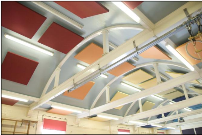
Sonata Vario installed to the ceiling Stanley Road Primary School, Worcester
